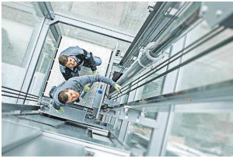
Dussmann Technical Solutions: Elevator technology
